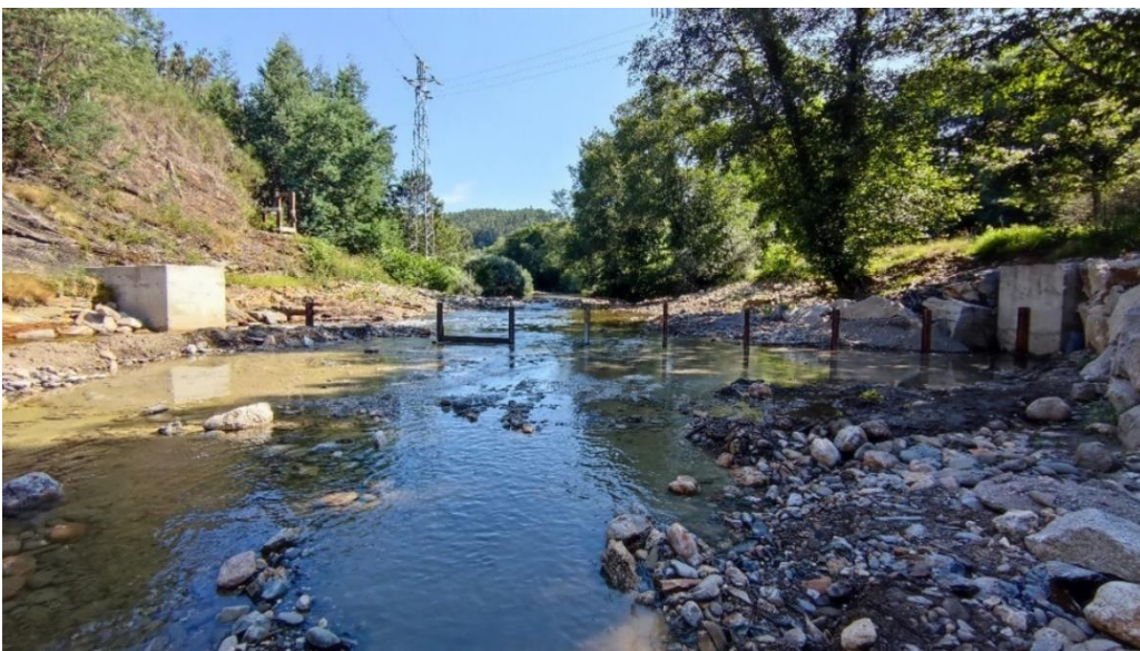
Figure 3 - Implementation actions: installation of a temporary weir and fish pass in River Águeda as part of the project's restoration works (action B1).
